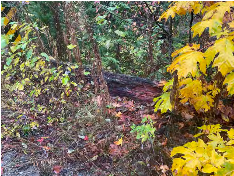
Downstream right bank fender extremely rotten
