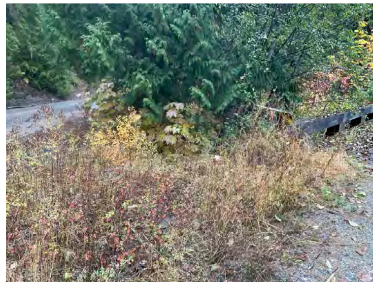
Missing downstream left bank fender
