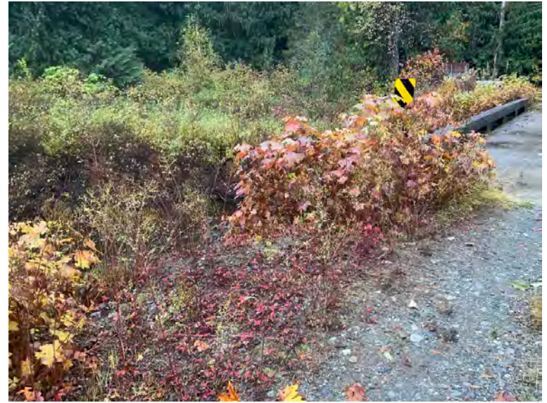
Missing upstream right bank fender
